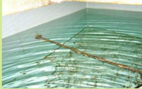
Light debris but corrosion to restraining bars
