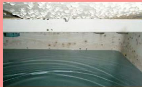
Gel coat (glass reinforced plastic) failure resulting in local biological fouling (dark spots)
